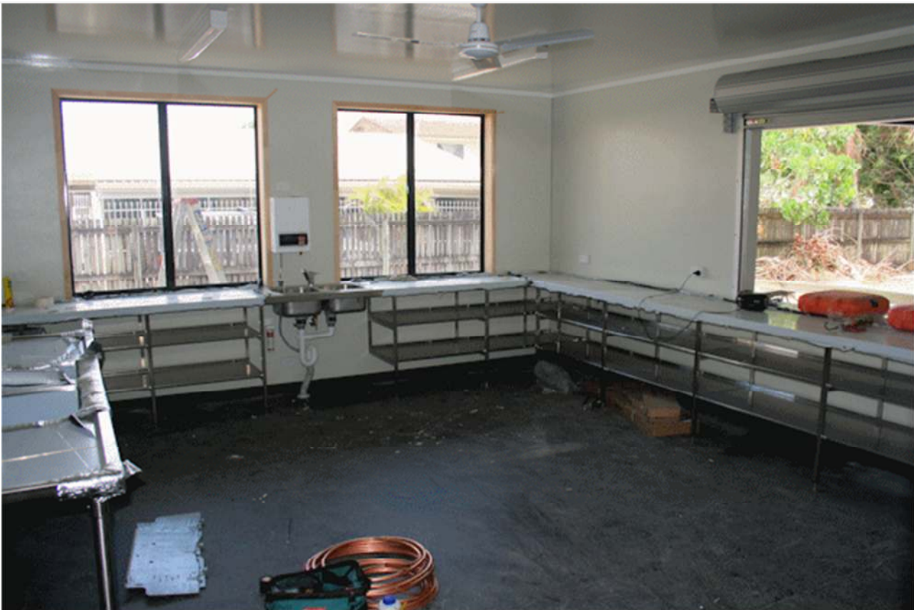
The stainless kitchen benches are all in. The walls will have stainless splashbacks installed next week.
